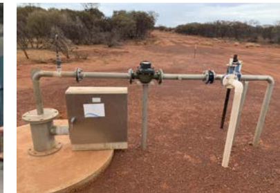
Sealed tanks and bores
