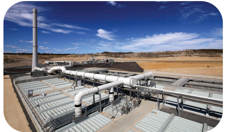
Figure 24: Alkimos WWTP odour control
