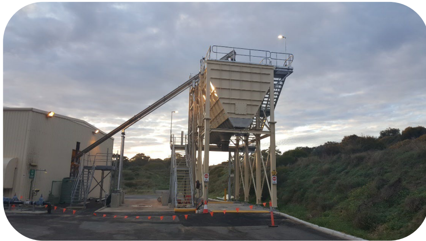
Figure 11: Bunbury sludge hopper
