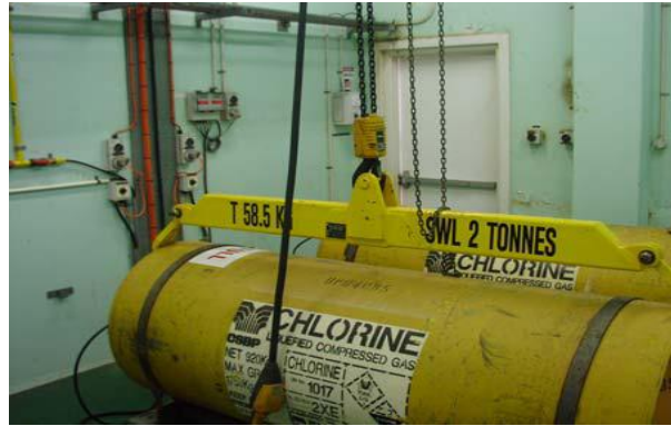
Typical drum lifting beam mounted on chlorine drum
